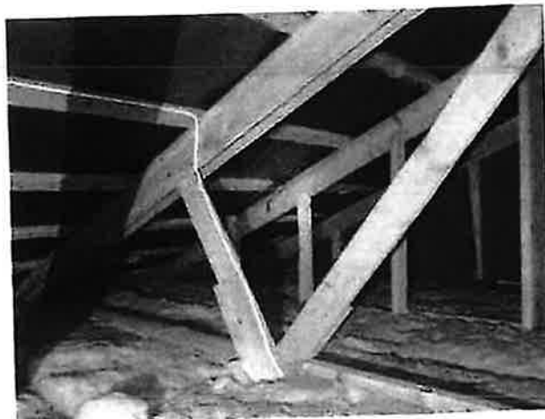
Fukt langs takstol i sone over bod.
